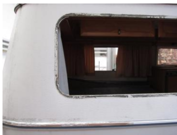
An overview of three possible weak points: roof sealing, window sealing and assembly weld upper to lower trailer body The reason here: old and porous window sealing
